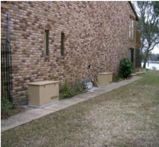
Two Generators on End of Building
