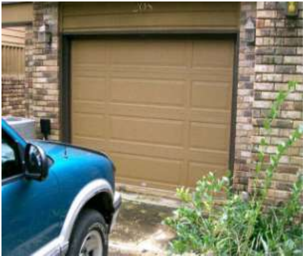
Unit 208 New Approved Door Unit
